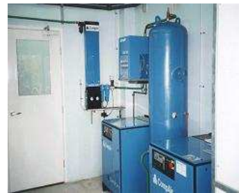
COMPRESSED AIR PREPARATION 压缩空气预备
